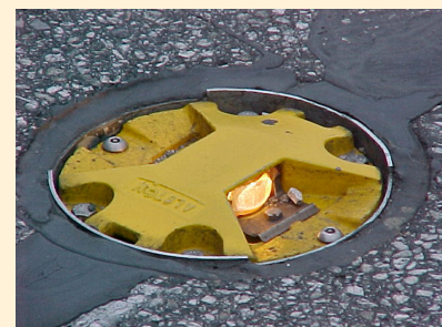
An in-pavement flashing warning light
