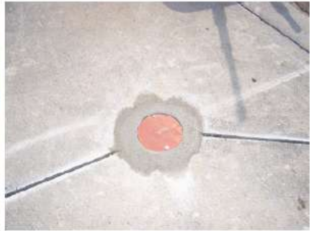
8. Plywood Protective Cover
