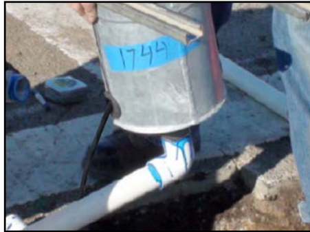
Base Can Attached to Drain Conduit
