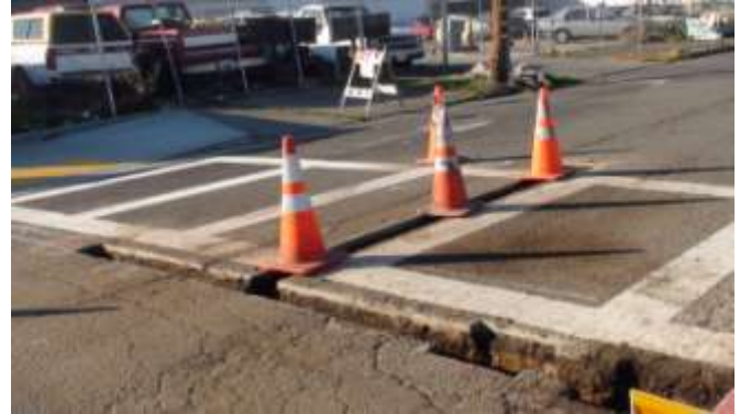
11. Trench is now completed and ready for Installing the Base Cans and Conduit.
