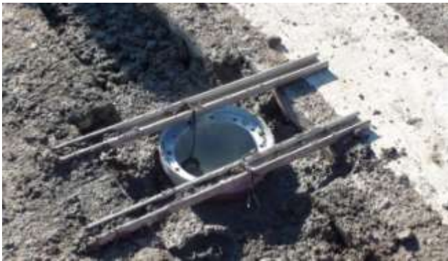
22. Quick dry concrete is generally used around the base cans; Standard concrete mix is used everywhere else.
