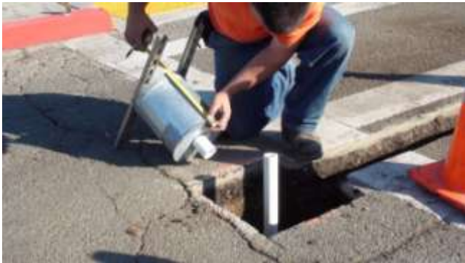
16. Base cans are then attached to drain conduit using the PVC fittings
