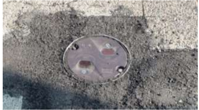
41. The plywood covers are then removed and replaced with fixtures. The fixtures are bolted to the base can. Silicon sealant is then placed into the space between the base can and fixture, providing a water proof seal.
