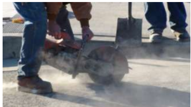
7. A dry cut is then made to cut along the outline of the trench.
