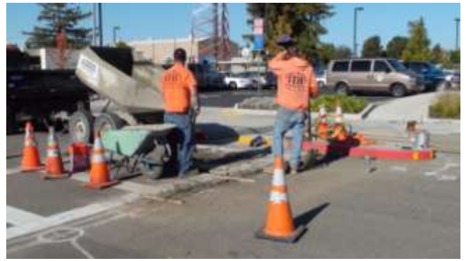
21. With all base cans, mounting jigs, drain and electrical conduit, and supports in place the concrete is poured and leveled.
