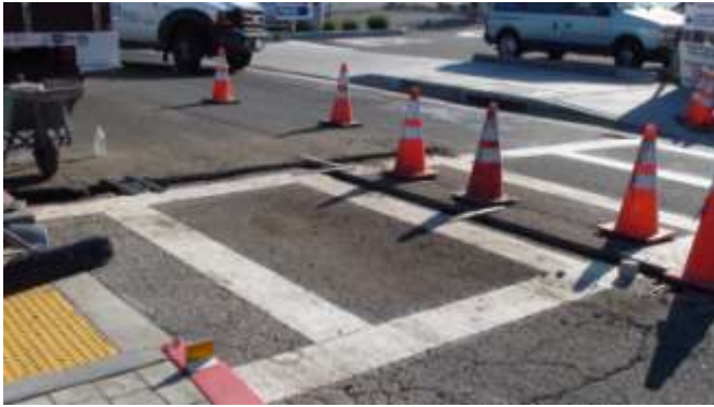
20. Wood stakes are put in place and attached to the electrical conduit with wire to support the conduit during the pouring of concrete.
