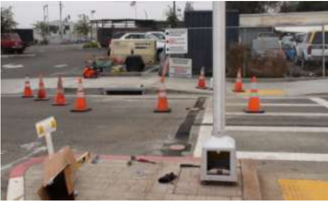
32. Pole and base are installed onto base foundation (base shown with access door open).
