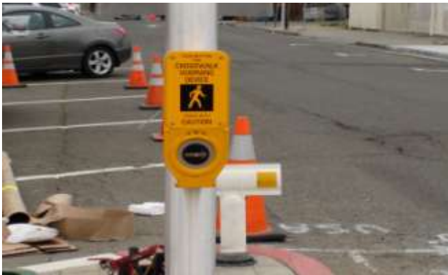
34. Cabling is attached to the terminals at the back of the pushbutton, and the pushbutton attached to the pole.
