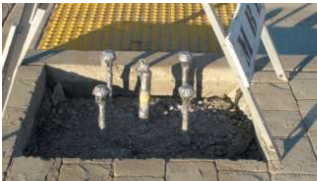
4. L-Bolts and electrical conduit are installed and a concrete foundation is poured at each pole base location.
