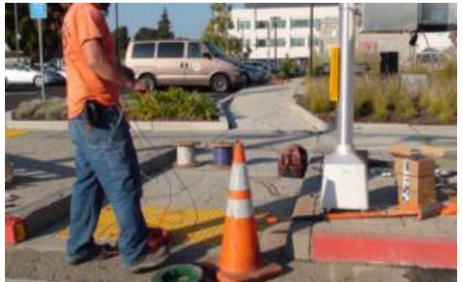
35. Infrastructure (street cabling) for fixtures, signs, and pushbuttons are measured and prepared for placement into the electrical conduit
