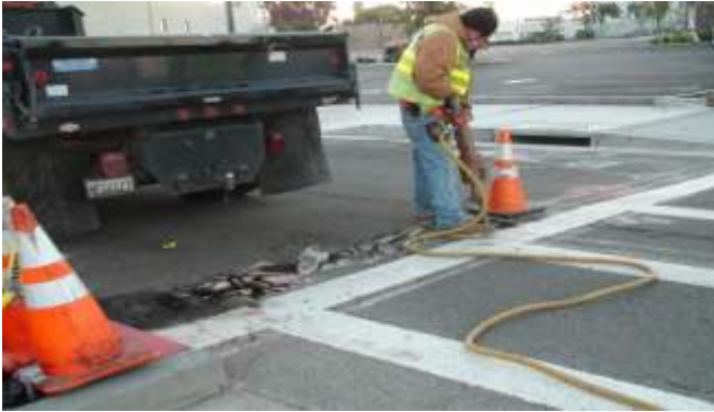
8. Next, a jack hammer is used to break-up the existing pavement within the trench.
