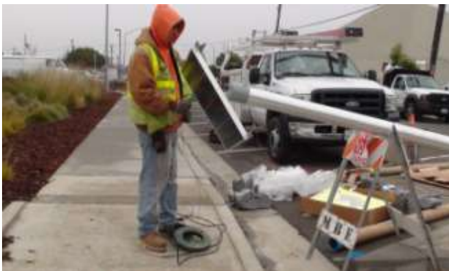
30. Using a steel tape, cabling is pulled through the inside of the pole and positioned to electrically connect system components.
