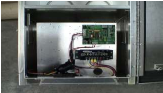
42. Final wiring is then made to the terminal block in the rear of the enclosure; the controller back panel is reinstalled, load and power cables connected, and the system's operating parameters set-up.
