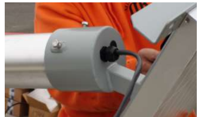
31. Waterproof fittings are installed on pole cap and cabling attached to the terminals inside the solar panel J-Box
