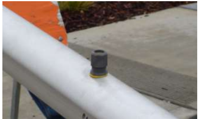
27. Waterproof Electrical Fittings are attached to the Pole for Flashing LED Sign Cabling.
