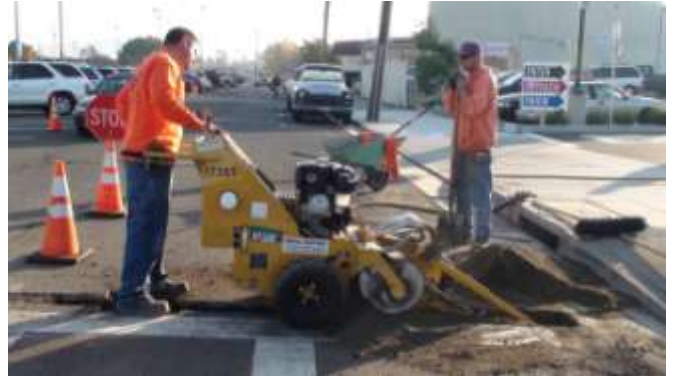
9. A trench digger is then used to remove pavement pieces and dig the trench.
