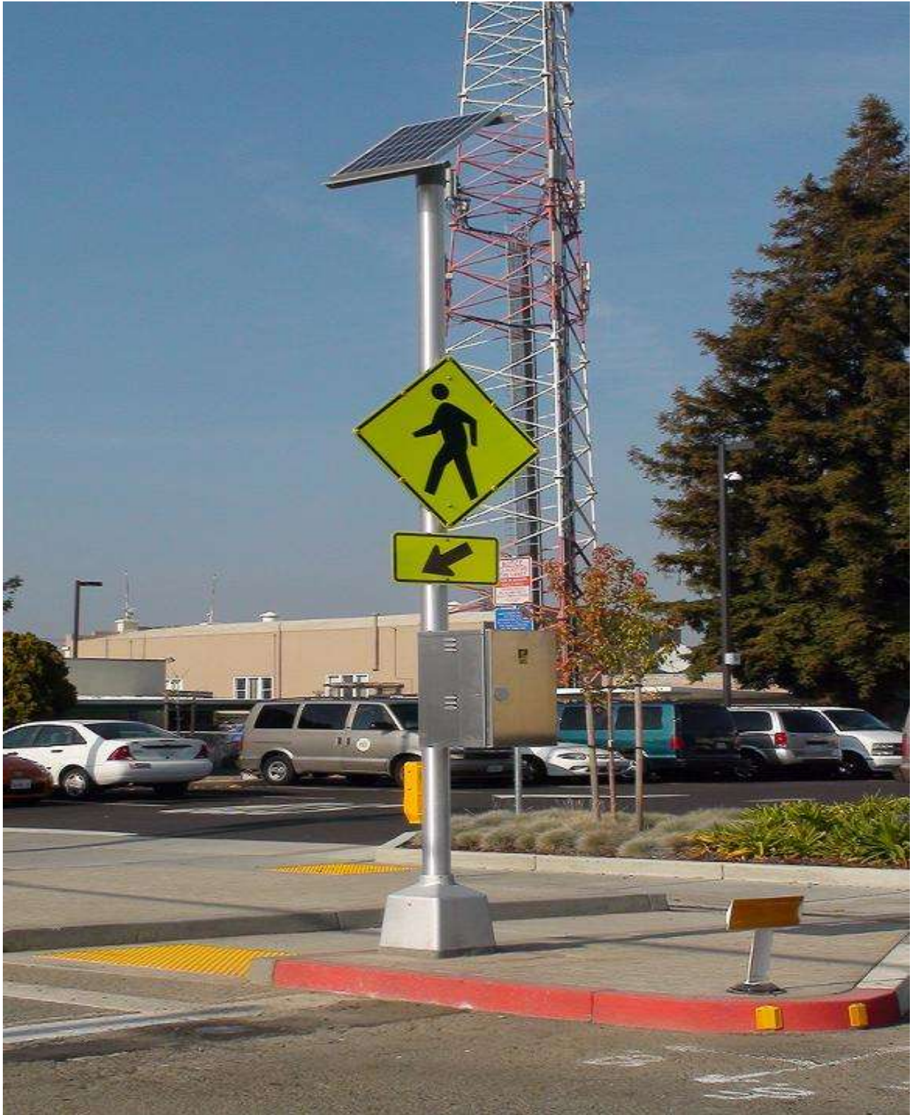
50. View of pole assembly showing the solar panel facing True South, the Flashing LED Pedestrian Sign, the Crosswalk Arrow Sign, and the TS1000 System Enclosure.
