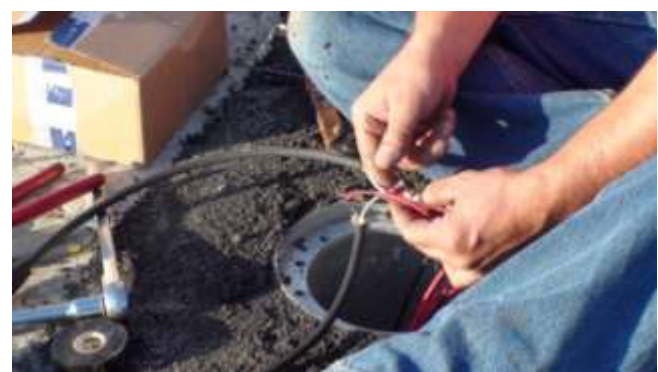
37. All cabling passes through the base cans. Fixtures are wired in parallel using water proof splices (white-to-red and black-to-black).
