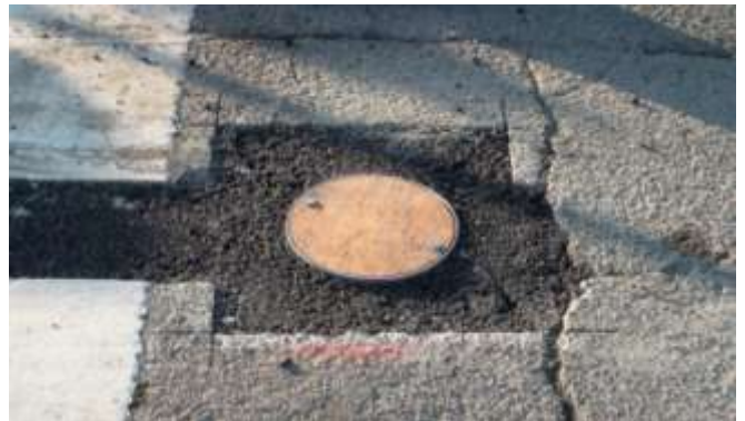
23. The mounting jig is removed, base can cleaned, and the protective plywood cover bolted onto the base can.
