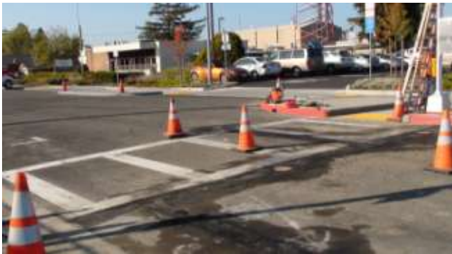
40. In-Pavement installation completed and ready for fixtures to be plugged into their connectors.
