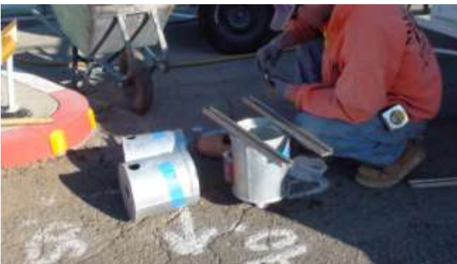
12. Base cans are fitted with a mounting jig (used to hold base can flush with road surface), and the conduit fittings attached to the bottom of the base.
