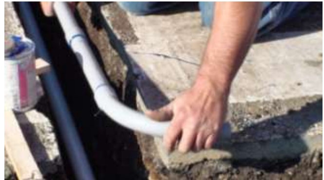
19. Electrical conduit is then installed above the drain conduit and connects with all base cans.
