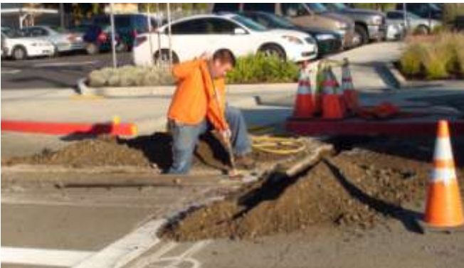
10. The final phase of the trenching is completed with the use of a trench shovel.
