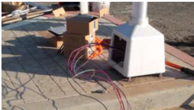
36. The process of passing the cabling through the base cans, to the pushbuttons and signs, and to the control system begins at the pole base.
