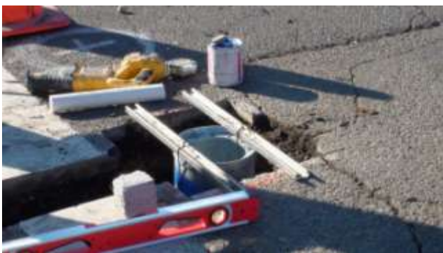
18. Dobie blocks are positioned under the conduit to prevent the base can from sinking after the mounting jig has been removed.
