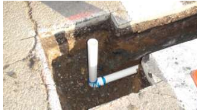
15. Drain conduit is positioned directly below the drain hole of each base can.
