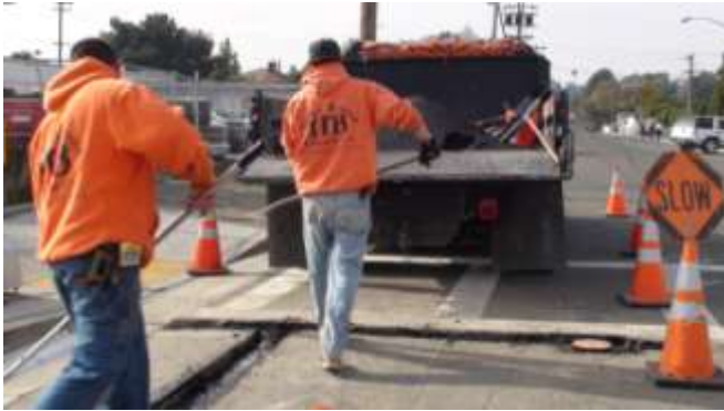
38. After all street cabling has been completed; asphalt is shoveled into the trench and leveled with a rake.
