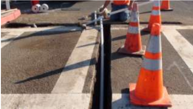
14. Drain conduit (PVC) is then installed between the base cans, and between base cans and the storm drain.
