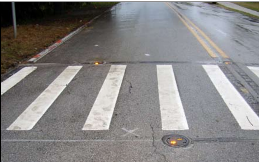
The solar-powered system of crosswalk lights flashing during activation.
